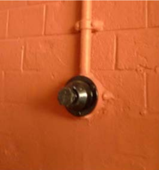
Heavy Duty Single Pol Rotary Switch at Old Peak School possibly from the General Electric Company of England.
